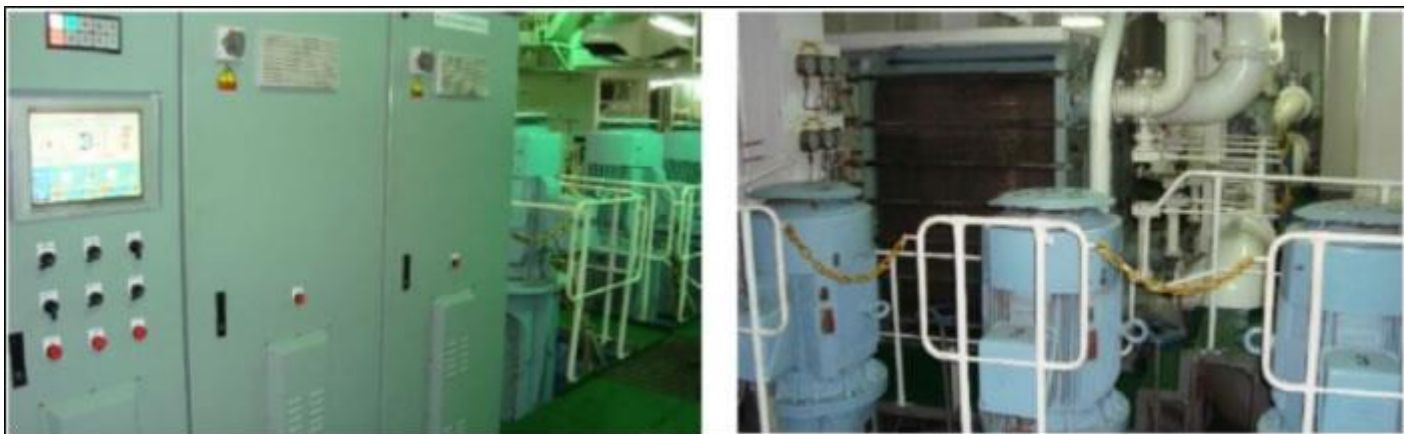
Figure 9 – Aspect of the SW circulation cooling pumps and respective Variable Speed Drives (left).
