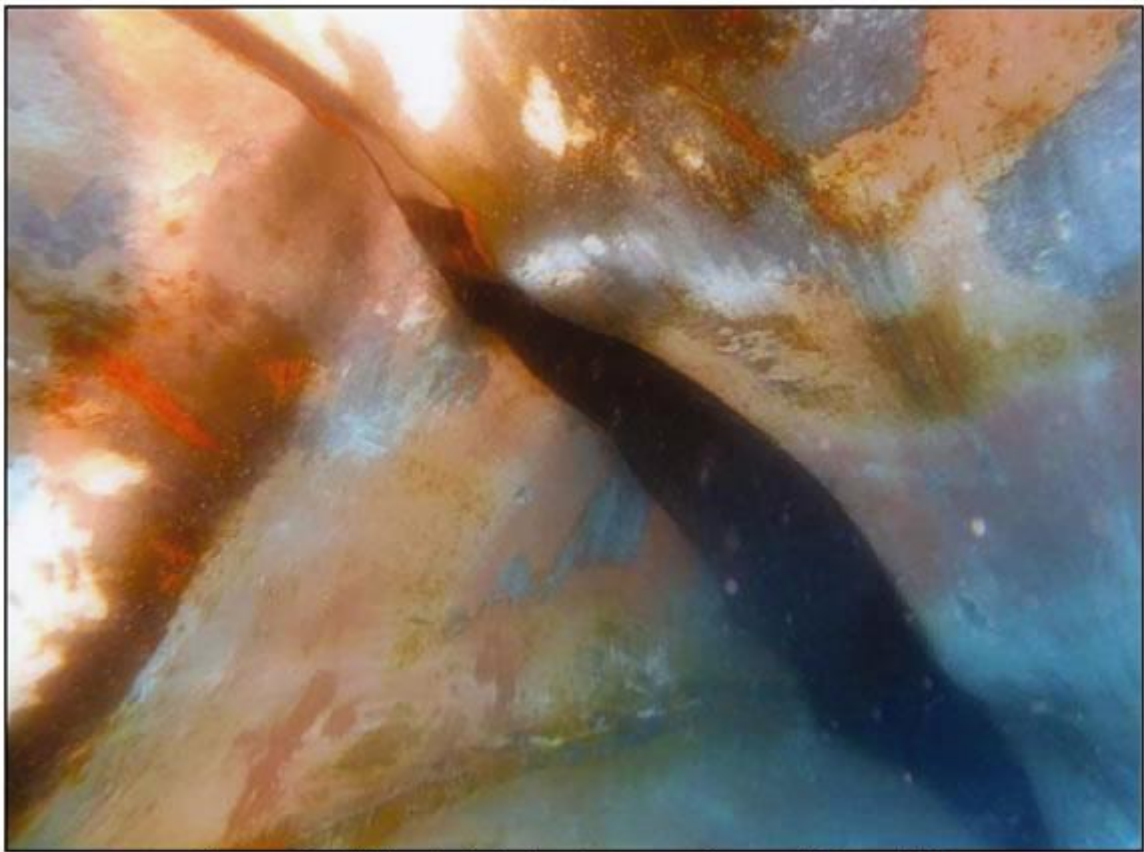
Figure 7: Split in shell plating between frames 169 and 178
