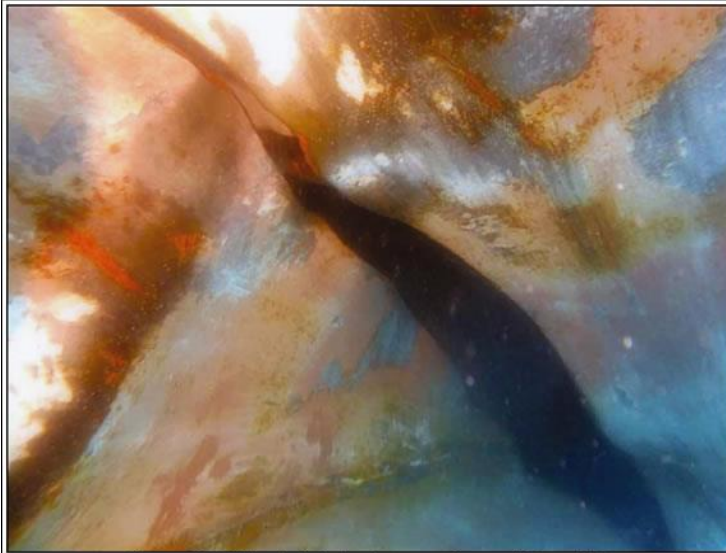
Figure 7: Split in shell plating between frames 169 and 178
