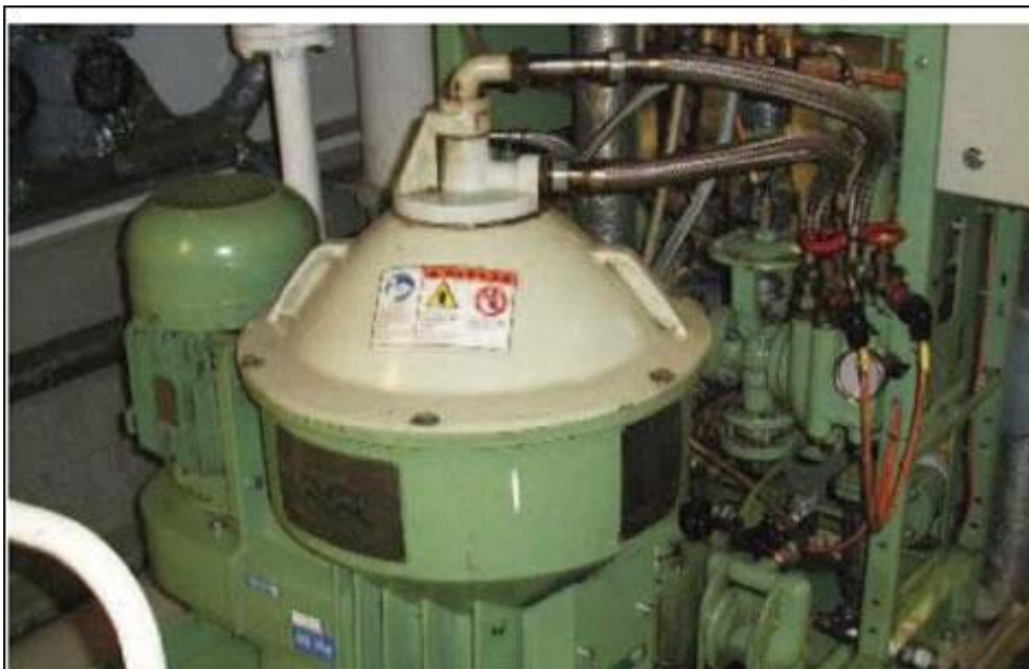
Lubricating oil purifiers extract solid and soluble impurities. Source: West of England.
