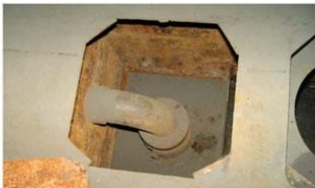
Hold suction arrangement and filter
