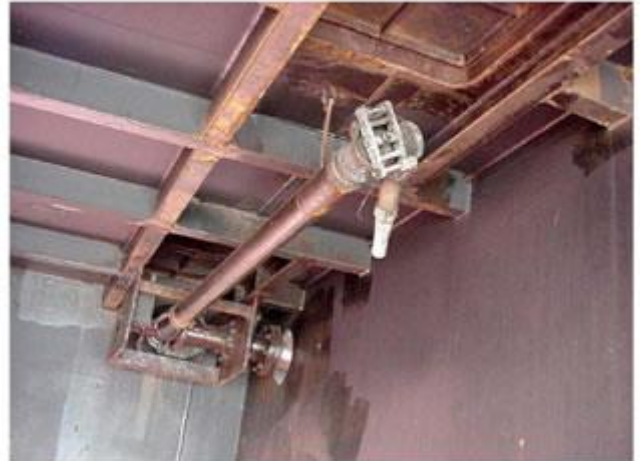
Fixed hold cleaning gun under hatch lids and fixed hold cleaning connection on deck
