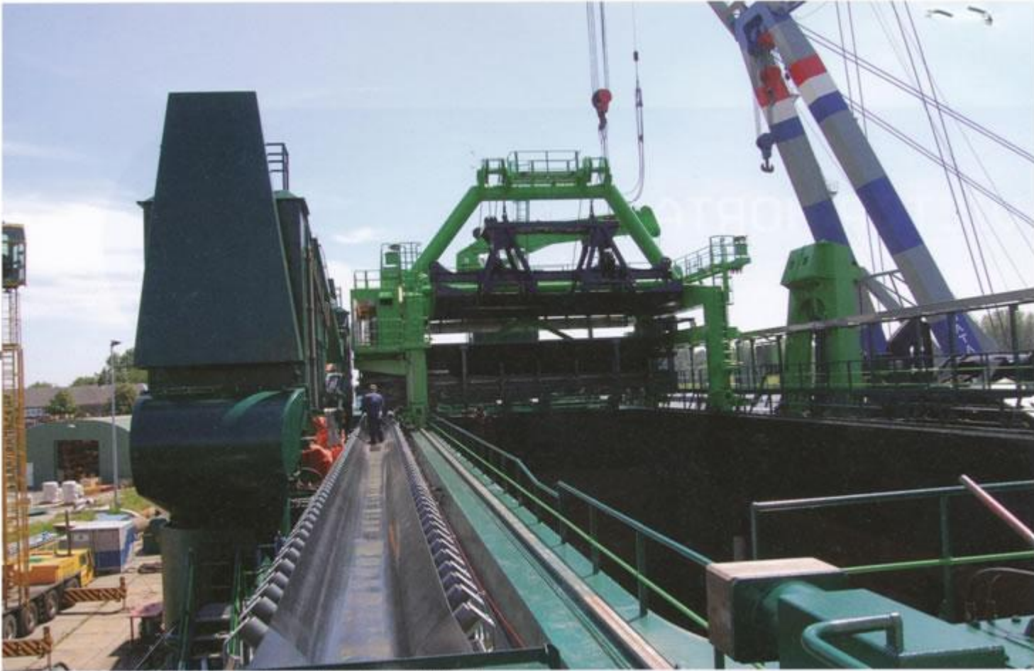
The screen towers can be rotated to make room for the travelling gantry crane with the grab
