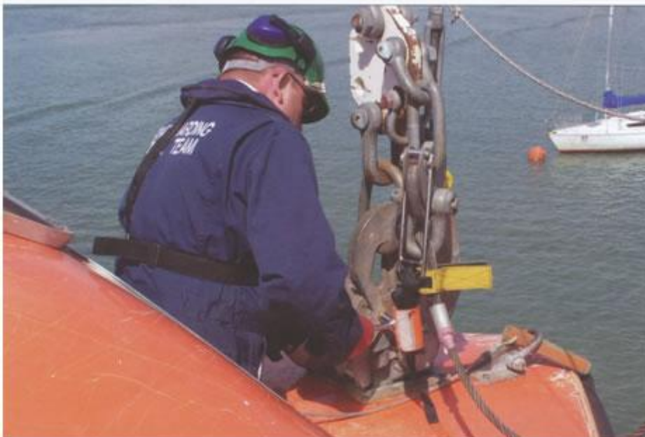
Schat-Harding engineer services a lifeboat hook
