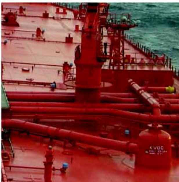
KVOC® drop pipe installed on Sallie Knutsen
