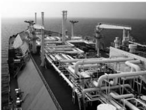
Fig. 5 Arrangement of piping on deck
